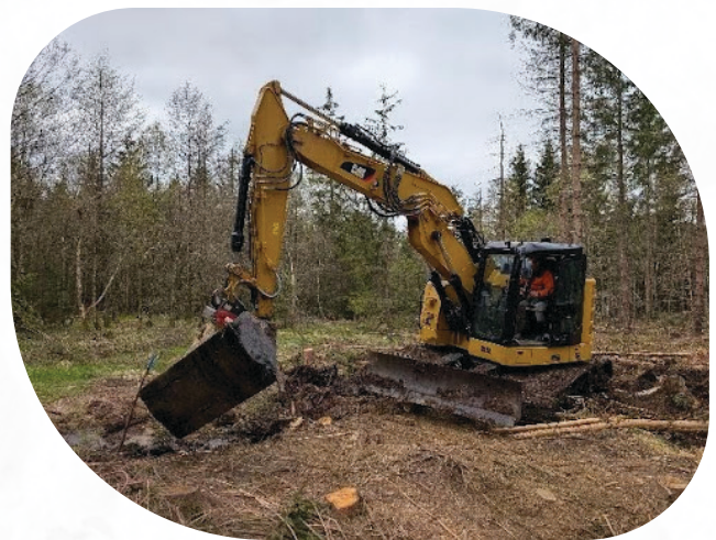
Figure 2. Implementation of restoration measures in the Klöckersfenn / Moorheide area. Upper picture: Aerial view after spruce removal and ditch blocking. Bottom: excavator works for the construction of ditch plugs. Machinery images: Stiftung Natur und Umwelt Rheinland-Pfalz (SNU).
